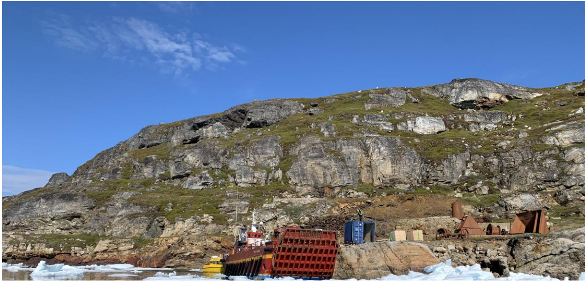
Figure 6: Drill Rig and equipment being unloaded to Amitsoq Island. Site of former graphite mine processing equipment on right. (taken 12 June 2021)
