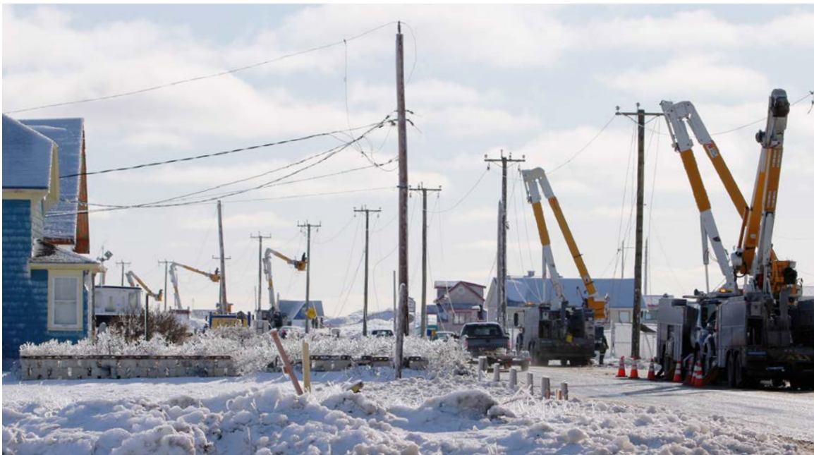
In February 2012, a severe ice storm seriously damaged the power system on the Îles de la Madeleine. Many line crews from across the province joined local teams to help restore service.
