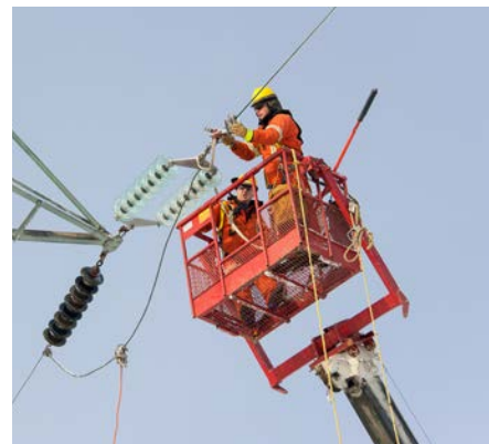
Line crew chief Réjean Morin and lineworker Guy Jr. Lavoie replace insulators on a 120-kV transmission line.
