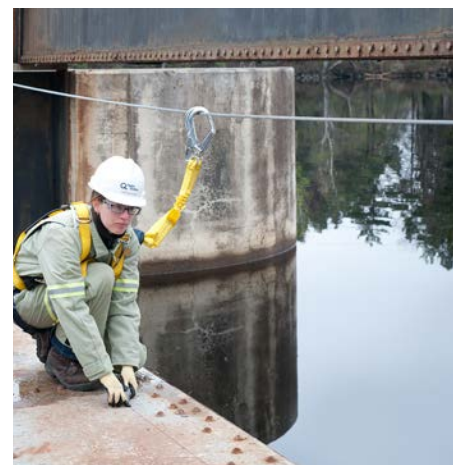
Civil engineering technician Stéphanie Cloutier inspects the gates of the Almaville spillway, one of structures in the Shawinigan complex.
