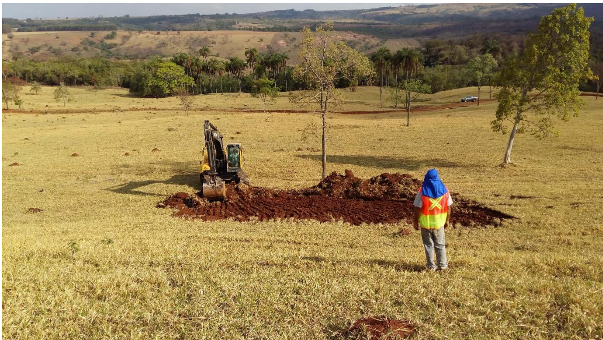
Figure 2: Excavator starting removal of topsoil in preparation of the commencement of opening pit mining
