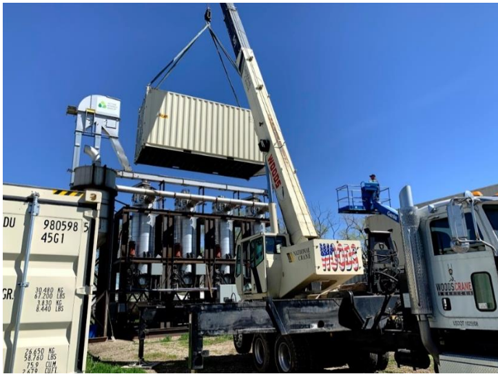
Figure 1: Disassembly of the plant at Utah ahead of transportation to the Lumberton Site
