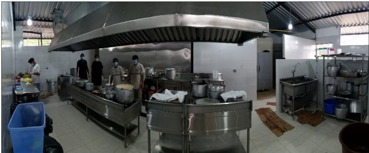
Figure 4: Alcala Base Camp facilities upgraded for the growing program at Cascabel.
