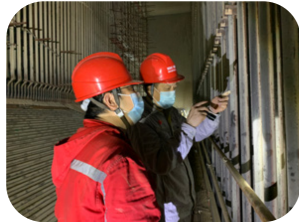
▲ SDIC Meizhouwan 3# "Four-pipe" inspection of the economizer, water wall, superheater and reheater inside the furnace
