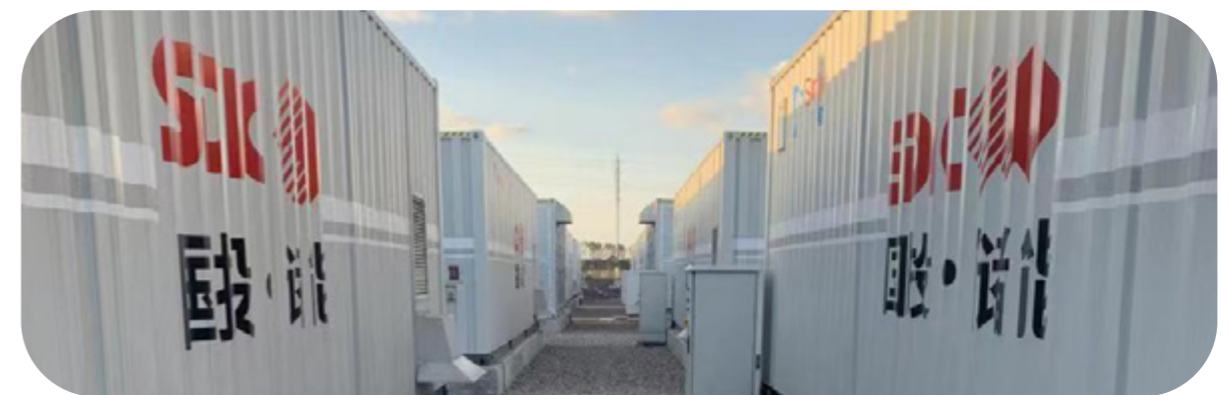
▲ Yancheng Zhihui Energy Storage Project put into operation
