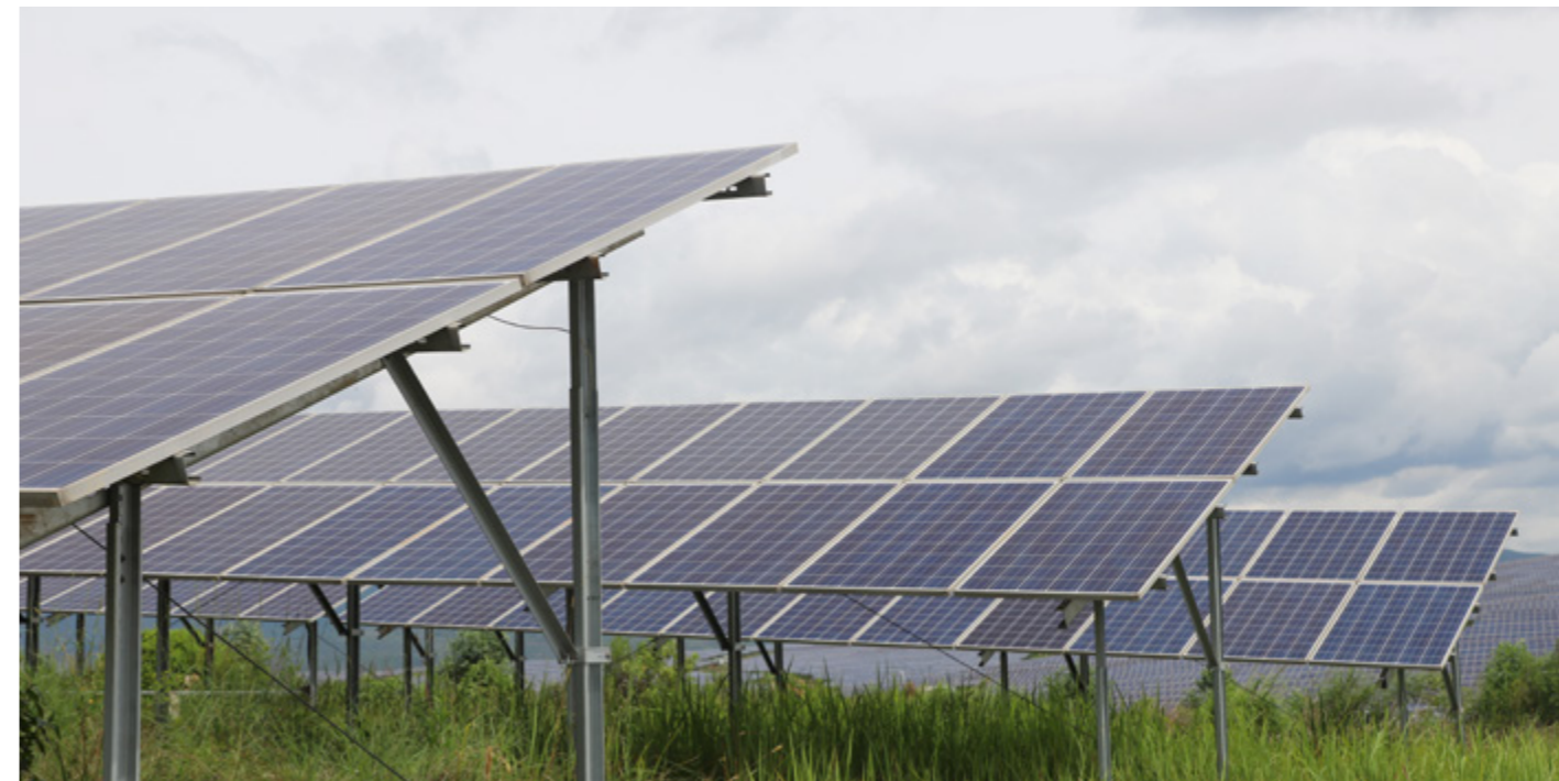
▲ SDIC New Energy · Honghe (Yunnan Nanzhuang solar power Project)
