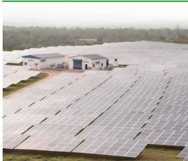
Solar park at Noamundi Iron ore mine
