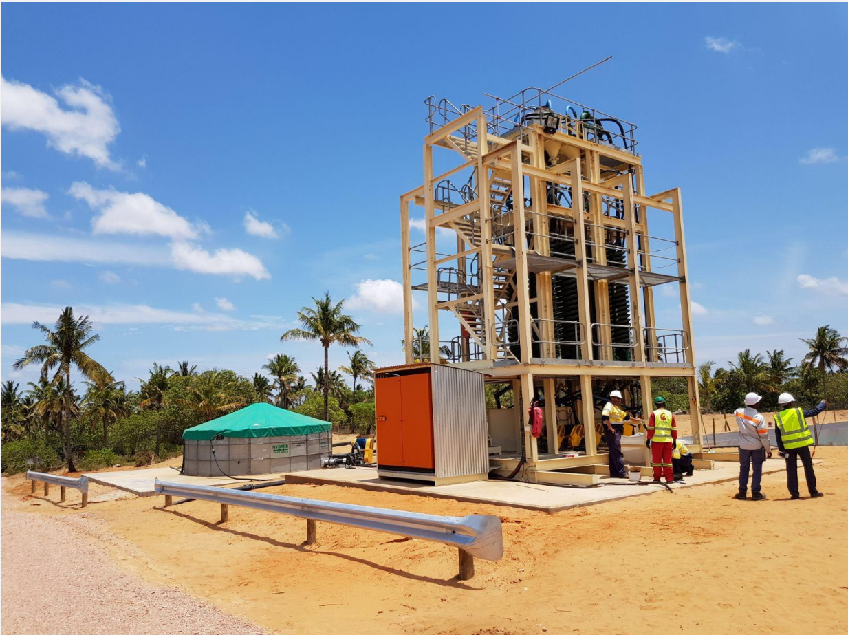
Figure 1. Photograph of plant at the Mutamba Project
