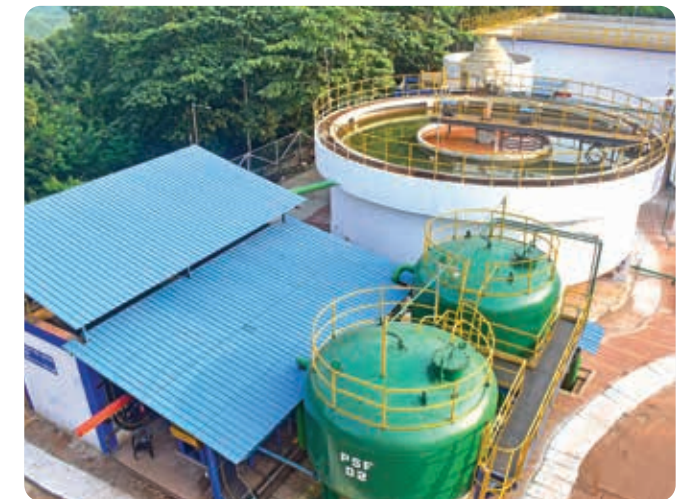
Water treatment plant at Noamundi, Jharkhand
