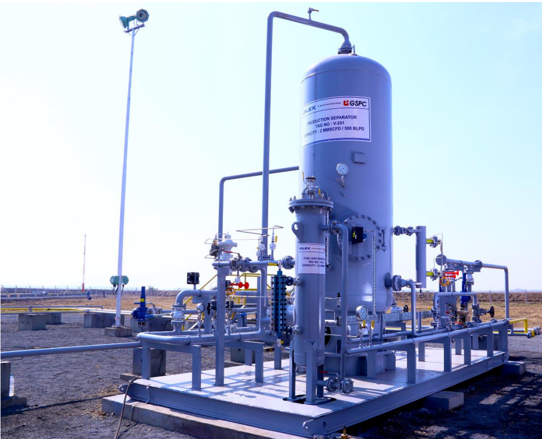
Figure 2 Separator, Bhandut Facility
