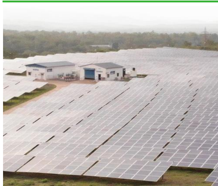
Solar park at Noamundi Iron ore mine
