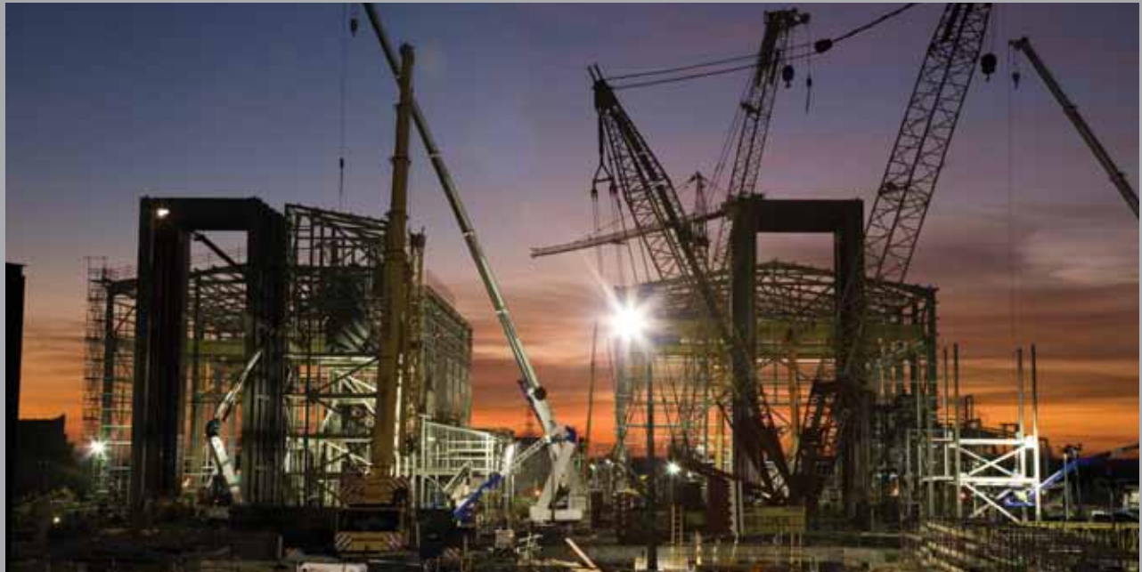
PROJECT → Staythorpe Power Station LOCATION → Newark
