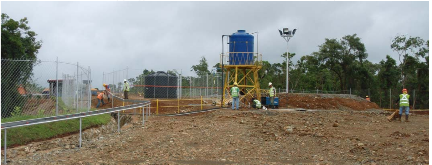
Fig 3 Acid makeup facility. Bunded Acid Tank (Black) and water tank (Blue) Hard stand area in foreground is where the 2m 3 per hour Resin in Pulp / Ion Exchange building is presently being constructed.
