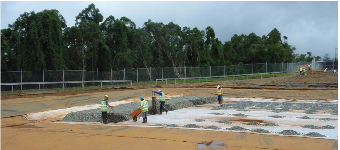
Fig 2 Heap leach Pad: Acid resistant pebbles being placed that form the base of the leach pad. Note Acid makeup area further up the hill to right of picture.
