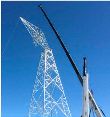
Chamouchouane–Bout-de-l'Île project: installation of the first tower in section 3, at Réservoir Taureau in Saint-Zénon (Mauricie region). Completion is slated for 2018.
