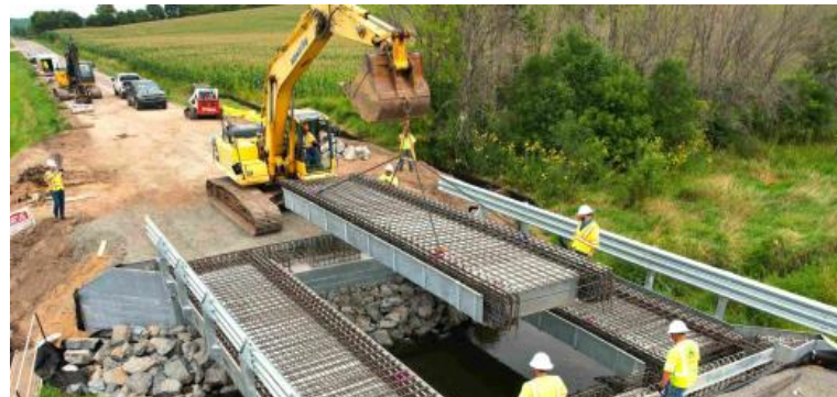
Successful execution of InQuik Bridge Proof of Concept project at Varanasi-Ranchi-Kolkata Expressway in record 24 days
