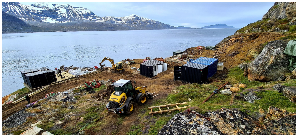
Figure 3. Installation of base camp at Amitsoq in readiness for start of phase 2 drilling (June 2022).
