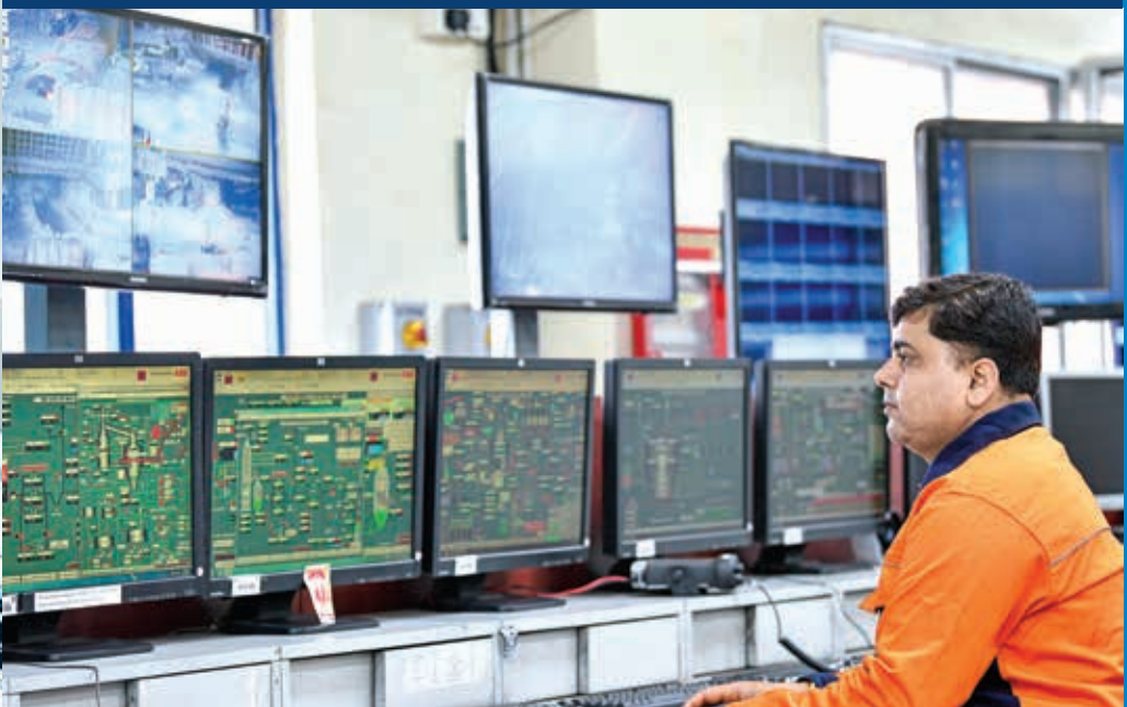
Control Room, Jamshedpur Steel Works
