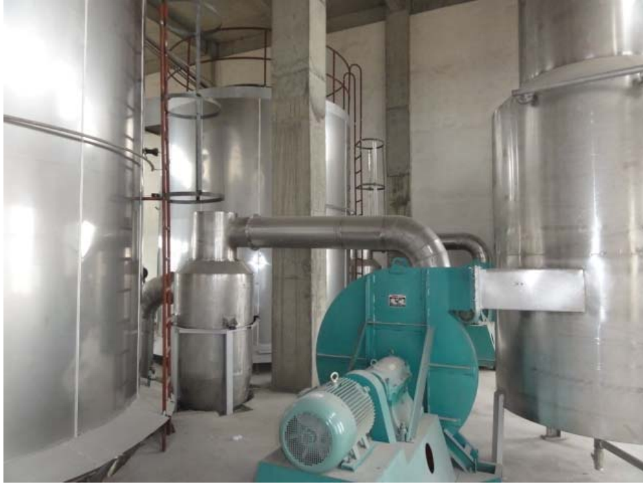
Machinery at new facility: November 2011
