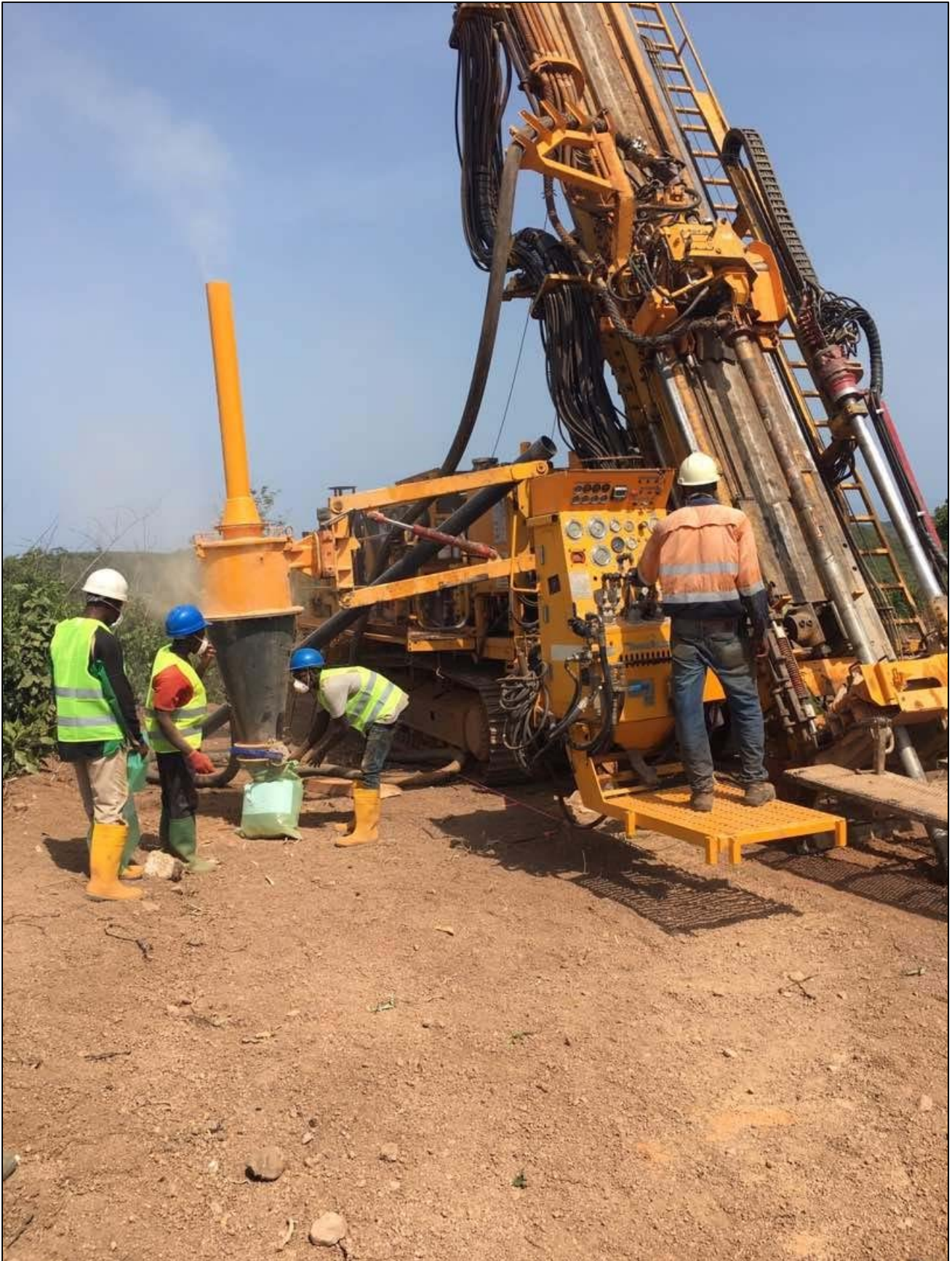
Photo: Geodrill multipurpose RC-DD rig collaring the first hole at the Ewoyaa lithium project
