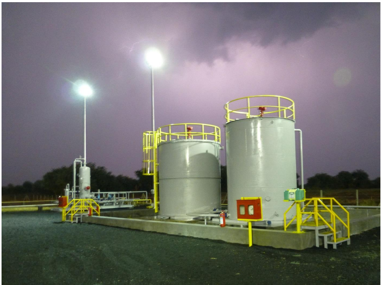
Cambay-73: Storage tanks
