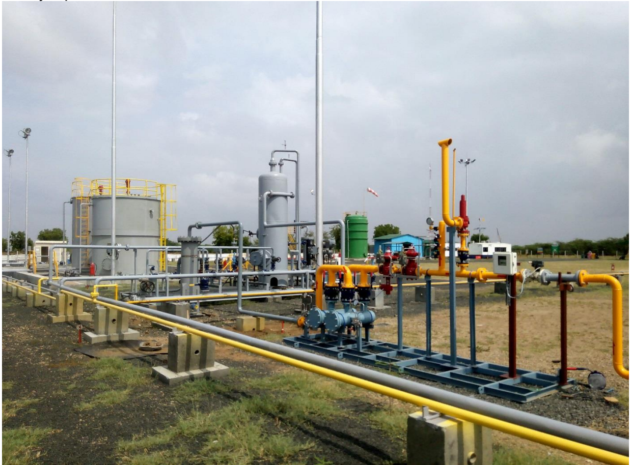
Cambay-73 production facilities
