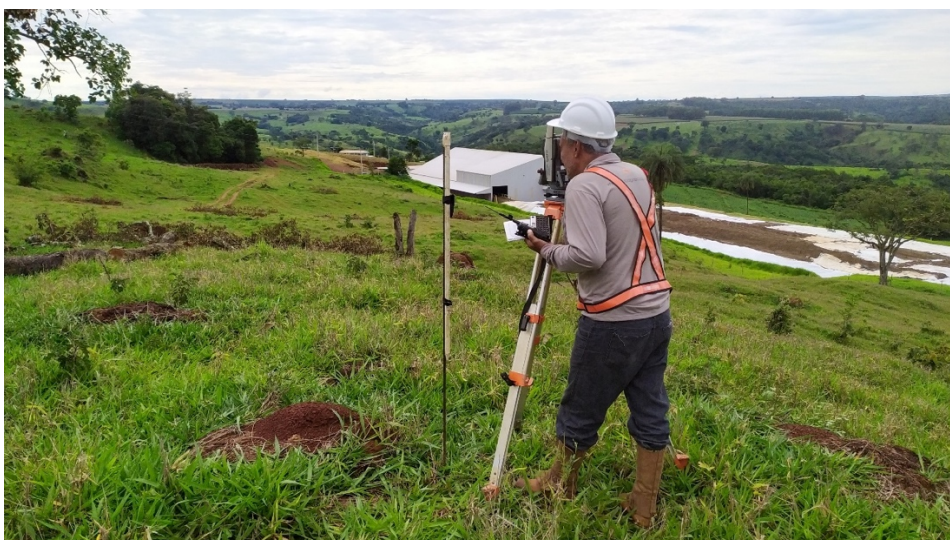
Figure 3: Surveying the location for the new ROM Storage area above the plant and existing ROM pads
