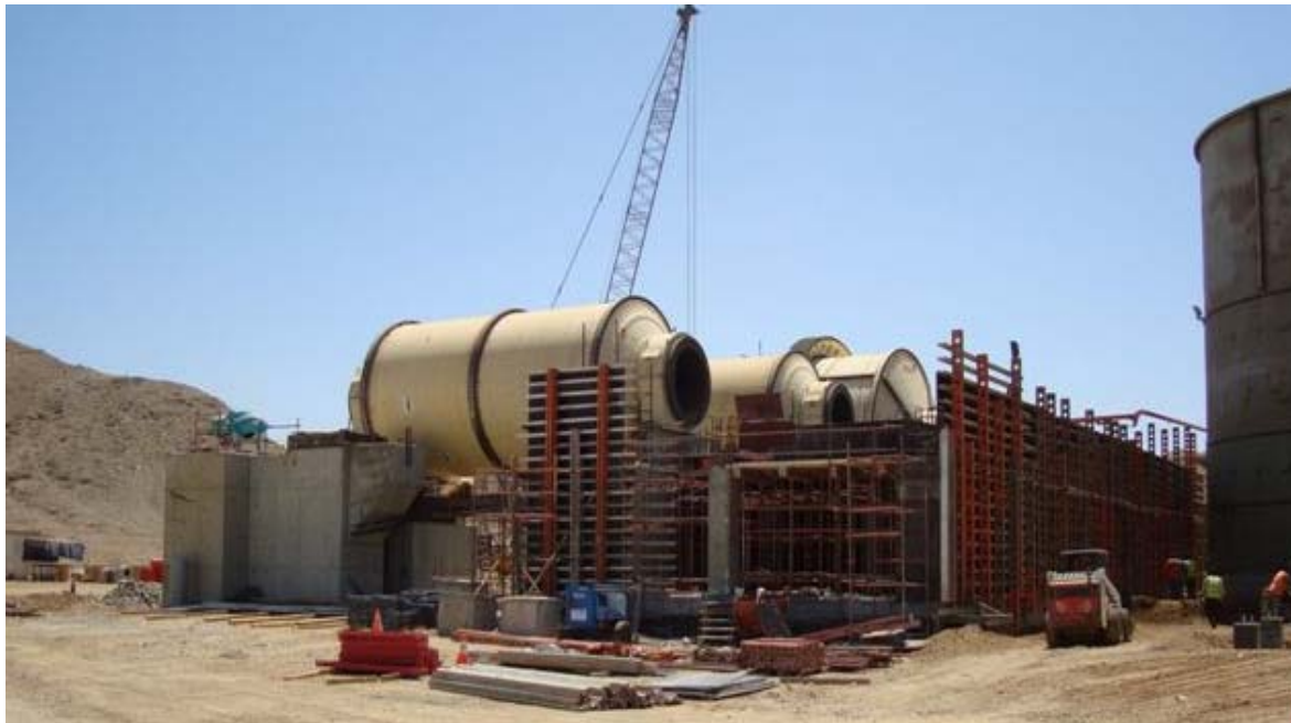
Progress Picture 1: Erection of MCC room underway (foreground) with Ball and SAG mills in place
