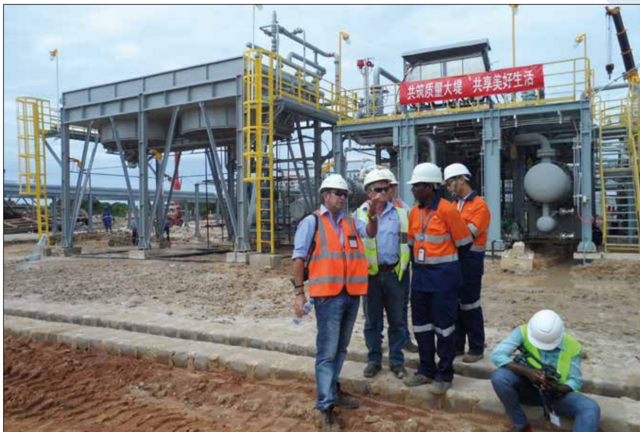
◆ New Songo-Songo processing plant
