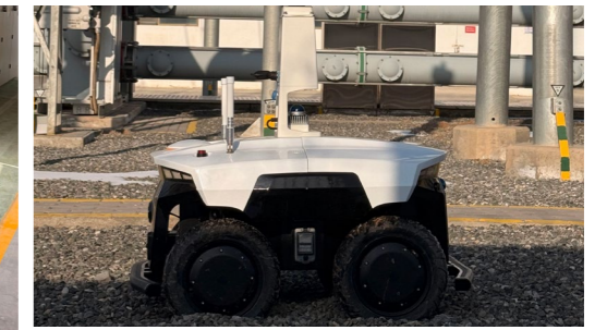
The wheeled outdoor robot inspects the equipment in the collection station
