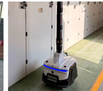
The wheeled indoor robot inspects the equipment in the high-voltage switchgear room
