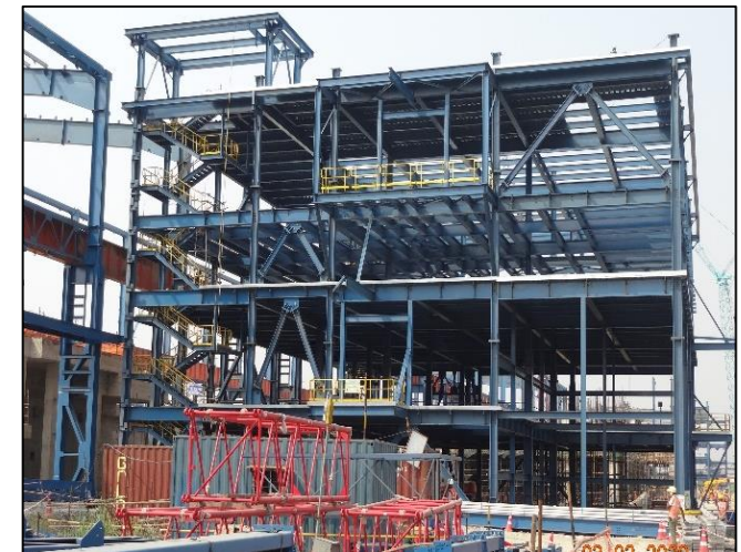
ECR Building of PLTCM
