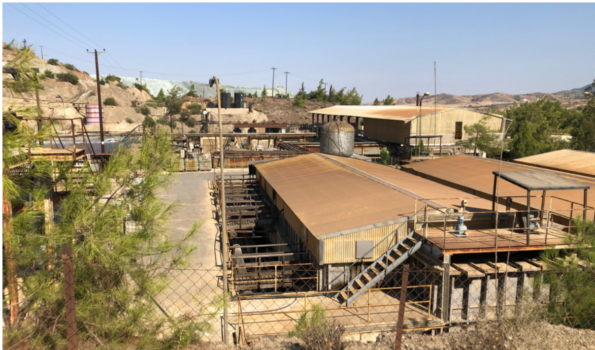
Figure 1: SX-EW processing plant installed at Skouriotissa as at 2019, which has since been dismantled by HCM ready for re-installation at Apliki. This processing plant was originally designed and built by Oxiana Limited (now Oz Minerals Ltd) in the 1990s and produced copper cathode from Skouriotissa for 24 years.
