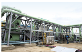
— Fugitive emissions process facility in semiconductor work sites
