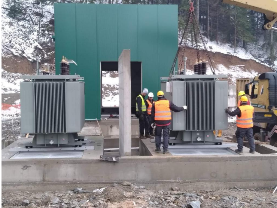
Figure 1: Rupice Transformer installation
