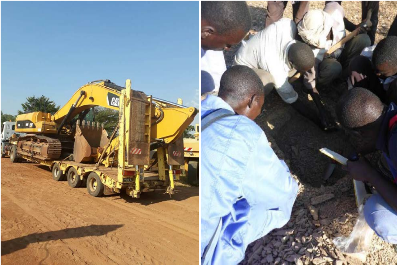
Figure 2 | Left: 30 tonne Excavator mobilised from N'Djamena to the Dorothe camp site. Right: Field training of soil sampling crews at Dorothe site
