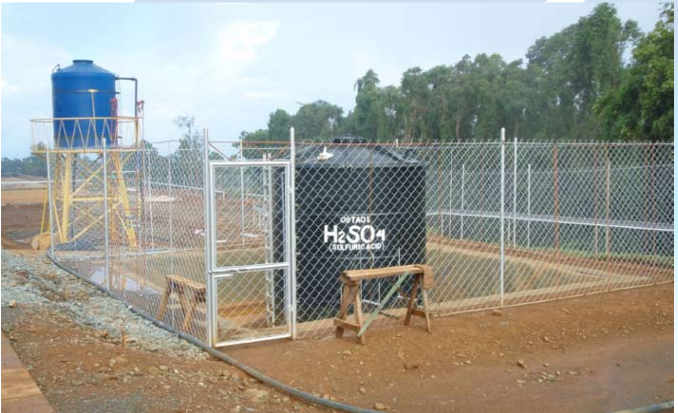
Acid and water tanks
