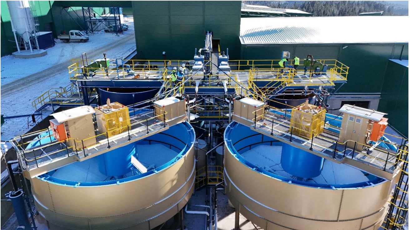
Figure 12: Thickeners (lead and zinc), January 2024
