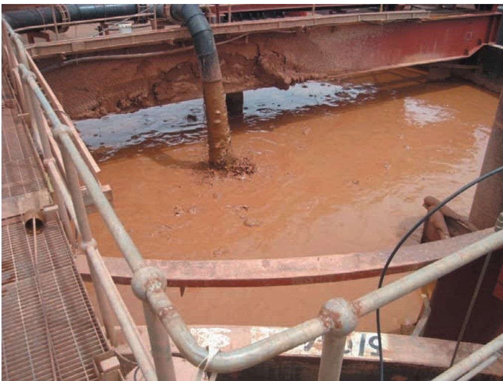
Photo 1.5: Thickened Feed Entering First CIP Tank
