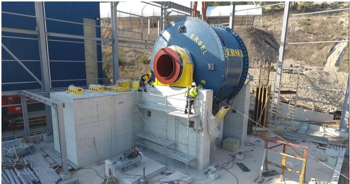
Figure 2: Installation of the new SAG mill at Kiziltepe, located in its final position, within the new mill building.
