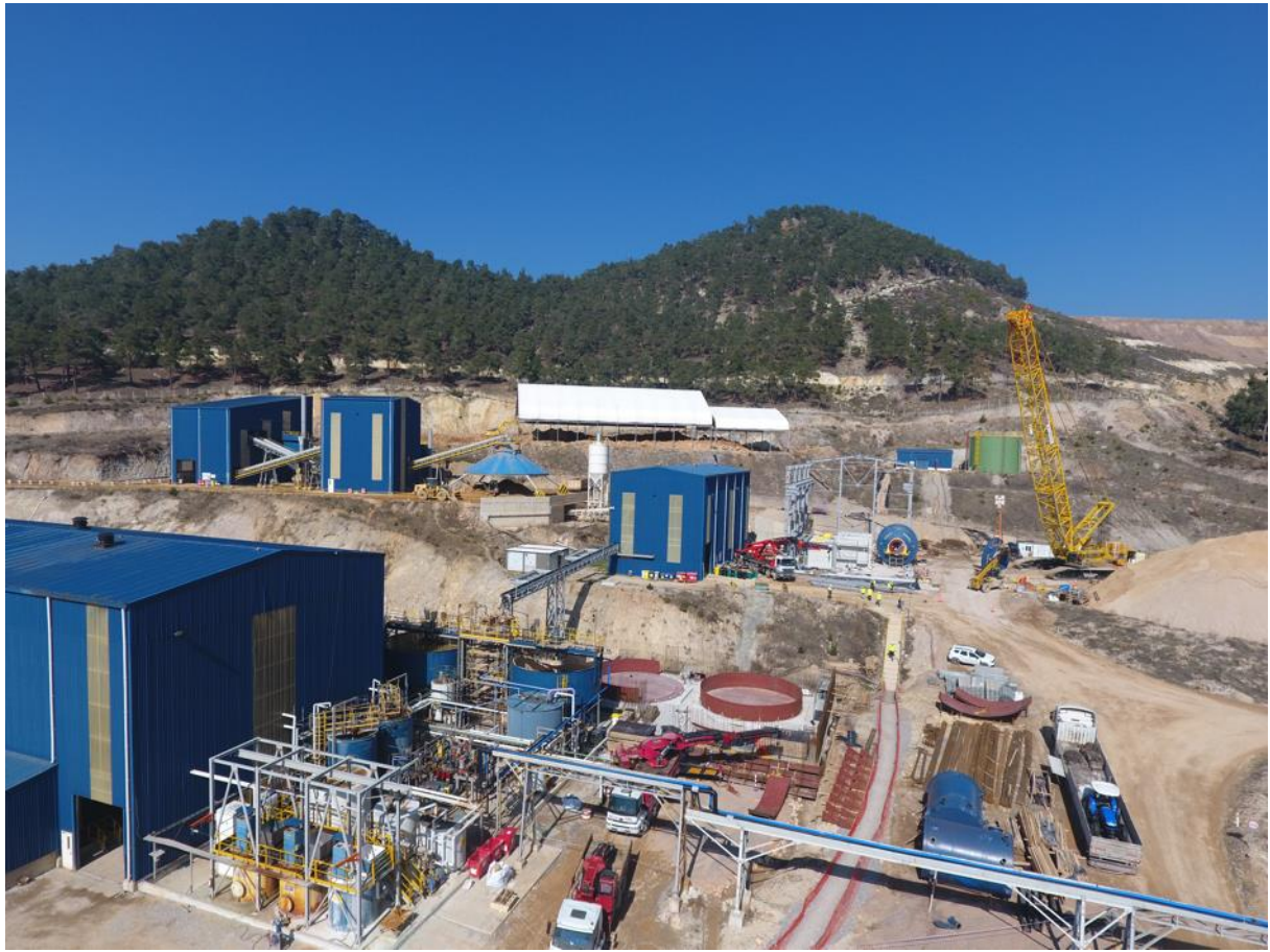
Figure 1: Processing plant expansion programme fully underway at Kiziltepe, with new semi-autogenous grind (SAG) mill about to be lifted by the crane into position, within the new mill building. In the foreground, additional pre-leach tanks are being constructed.
