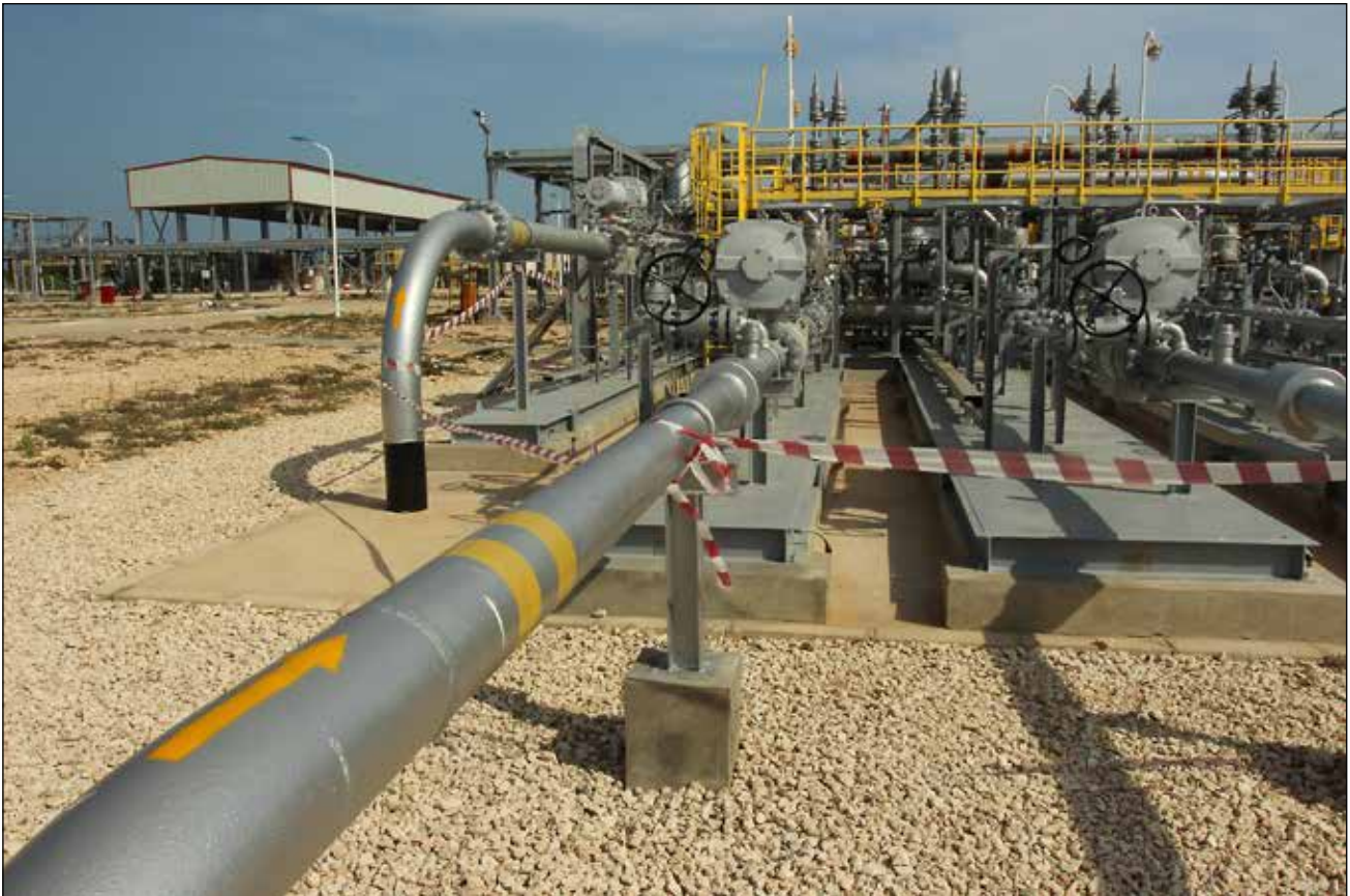
◆ KN-1 feed line into Songo Songo Island Gas Processing Plant
