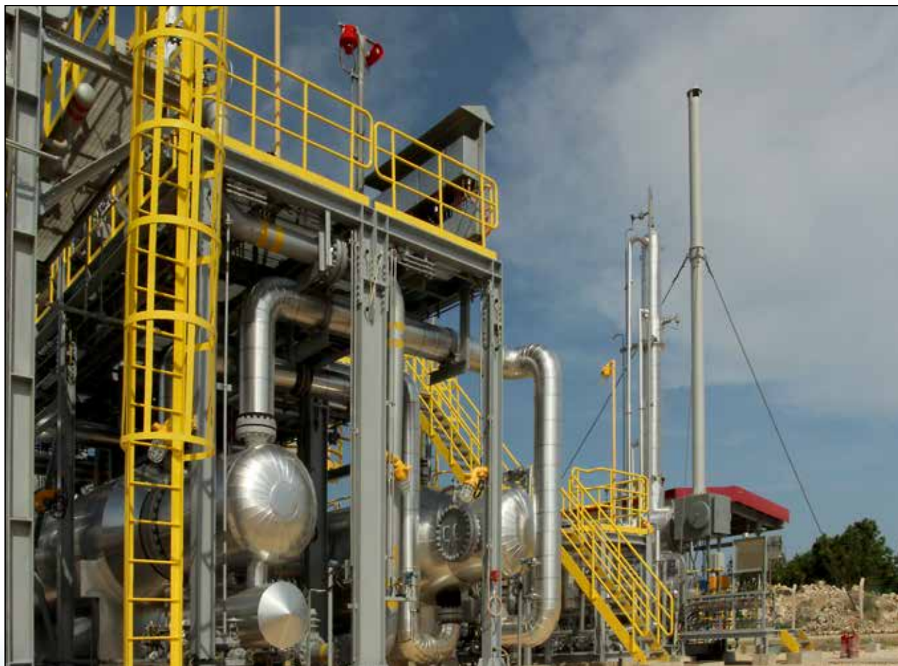
◆ Songo Songo Island Gas Processing Plant
