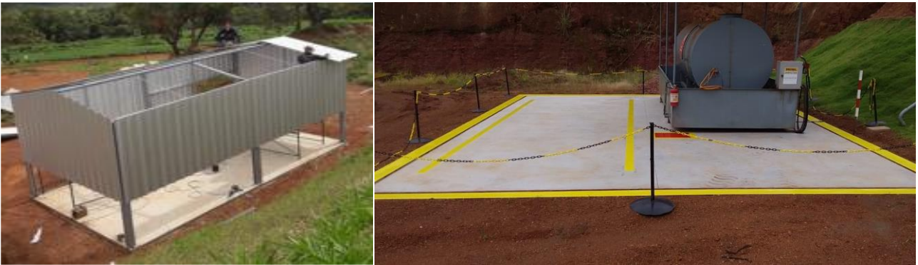
Figure 1: New trash storage facility and improved fuel storage area as required by environmental department as part of award of full mining permit.
