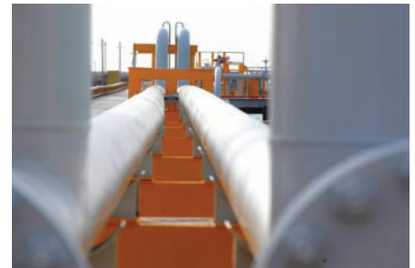
Above: Export lines to Aladja jetty.
