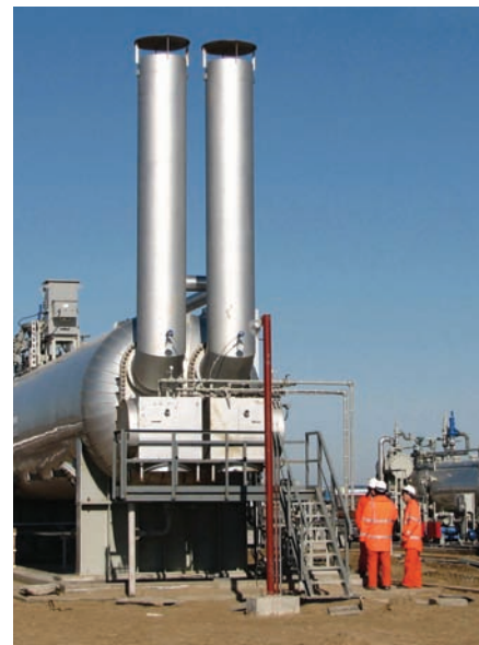
Above: Equipment at CPF.
