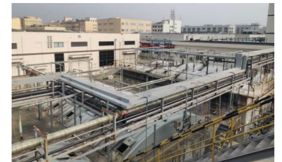
Wastewater Treatment Facilities
