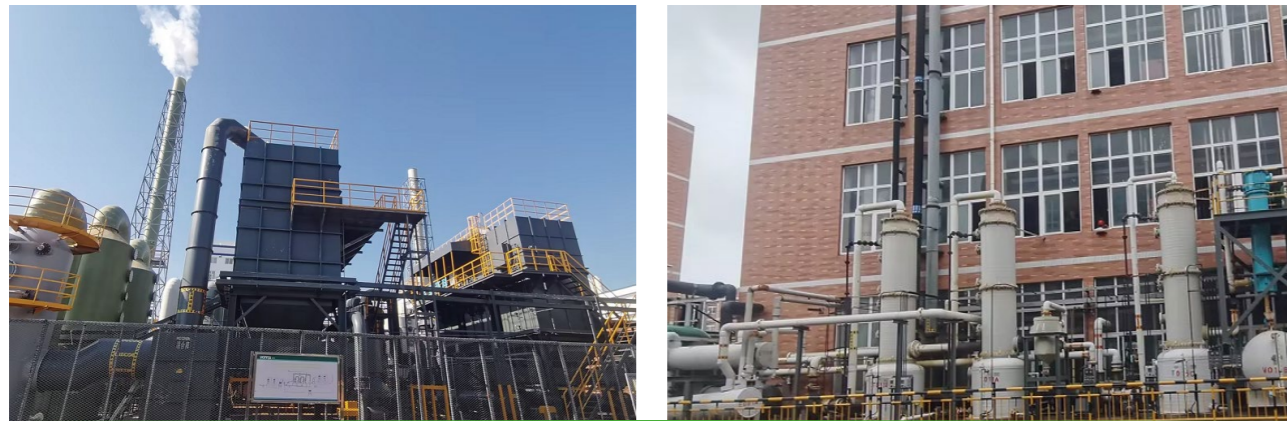
Waste Gas Treatment Facilities
